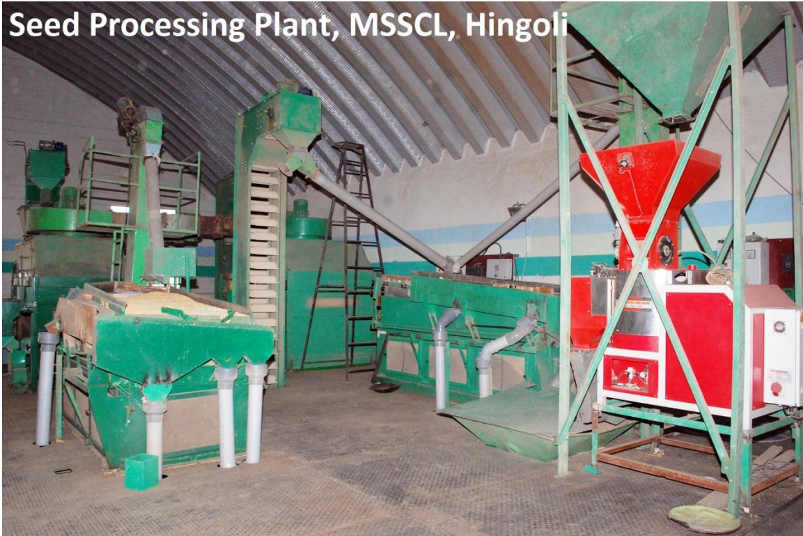
Seed Processing Plant, MSSCL, Hingoli
